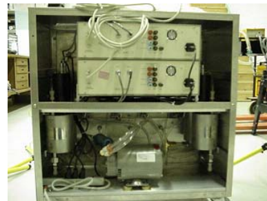
Bubblers and controls
